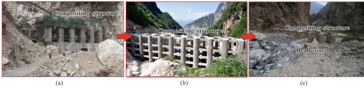
Fig. 45. Structural debris avalanche prevention in the transition zone: (a) Under construction; (b) Defense on debris avalanche; and (c) Arch effect to energy dissipation.
